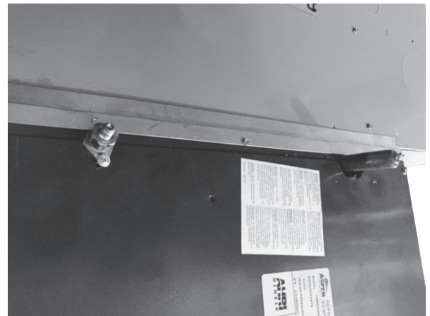
Top View of Cabinet
